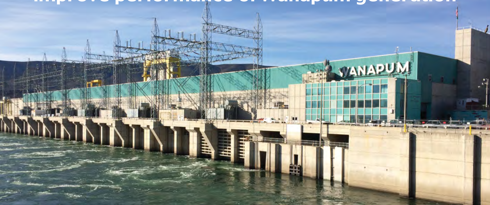
Wanapum Dam's SCADA systems give operators better control over power generation equipment. Photo provided by Grant County PUD.
