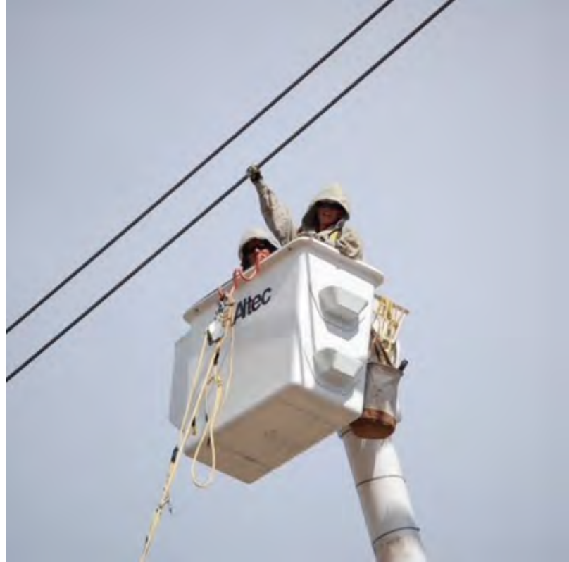
POWER's Sara Schroeder safely works on an energized line wearing a conductive suit and bonded to the conductor.
