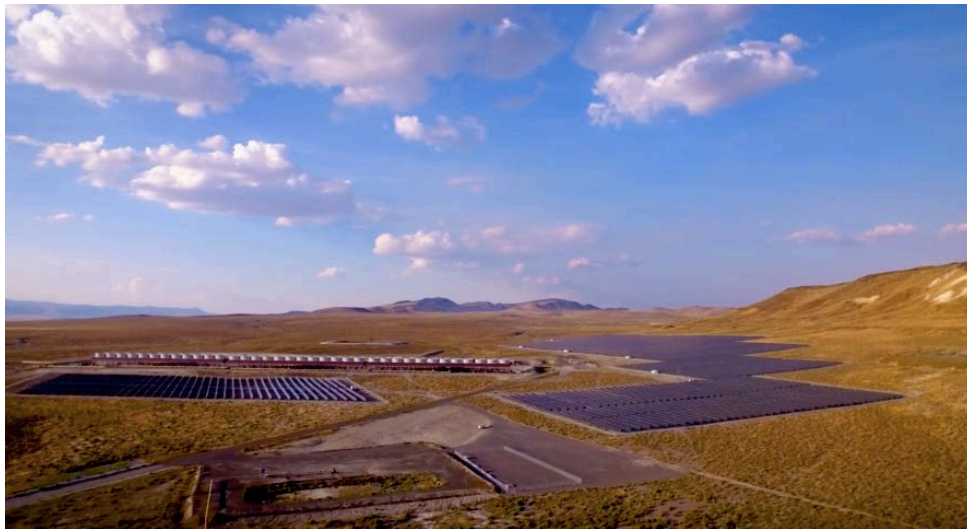
Patua geothermal plant with 10 MW solar PV field (ThinkGeoEnergy 2017)
